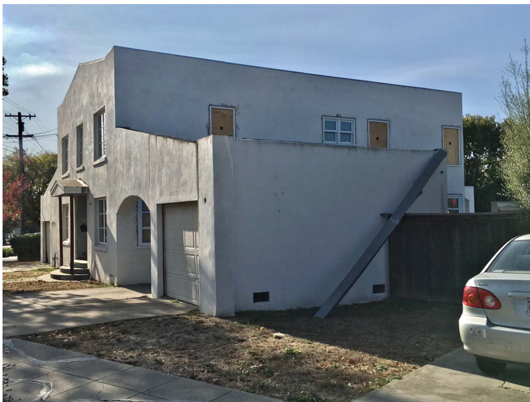
Figure 7: Larry Hickman's property, Nov. 19, 2019. These windows have been removed and replaced countless times, according to our neighbors. The gutter has been hanging off the wall since the end of October.
