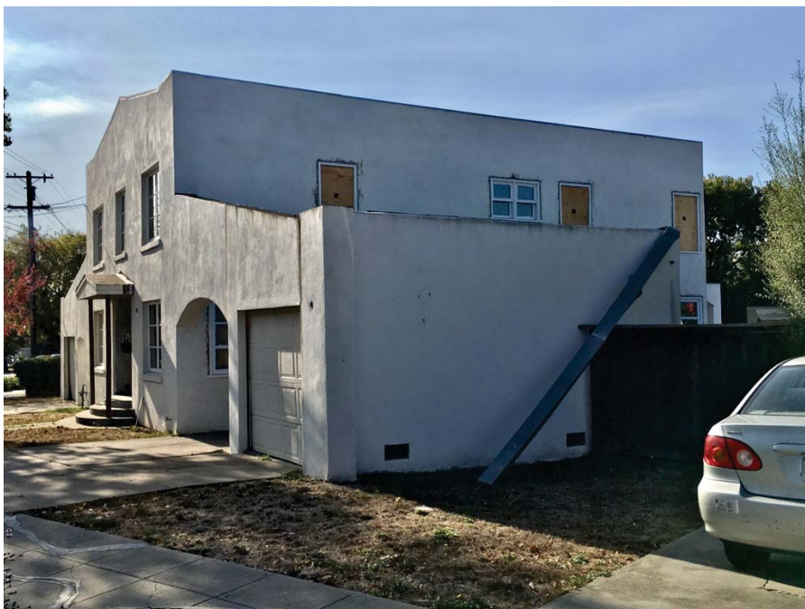
Figure 7: Larry Hickman's property, Dec 4 th , 2019. These windows have been removed and replaced countless times, according to our neighbors. The gutter has been hanging off the wall since the end of October.
